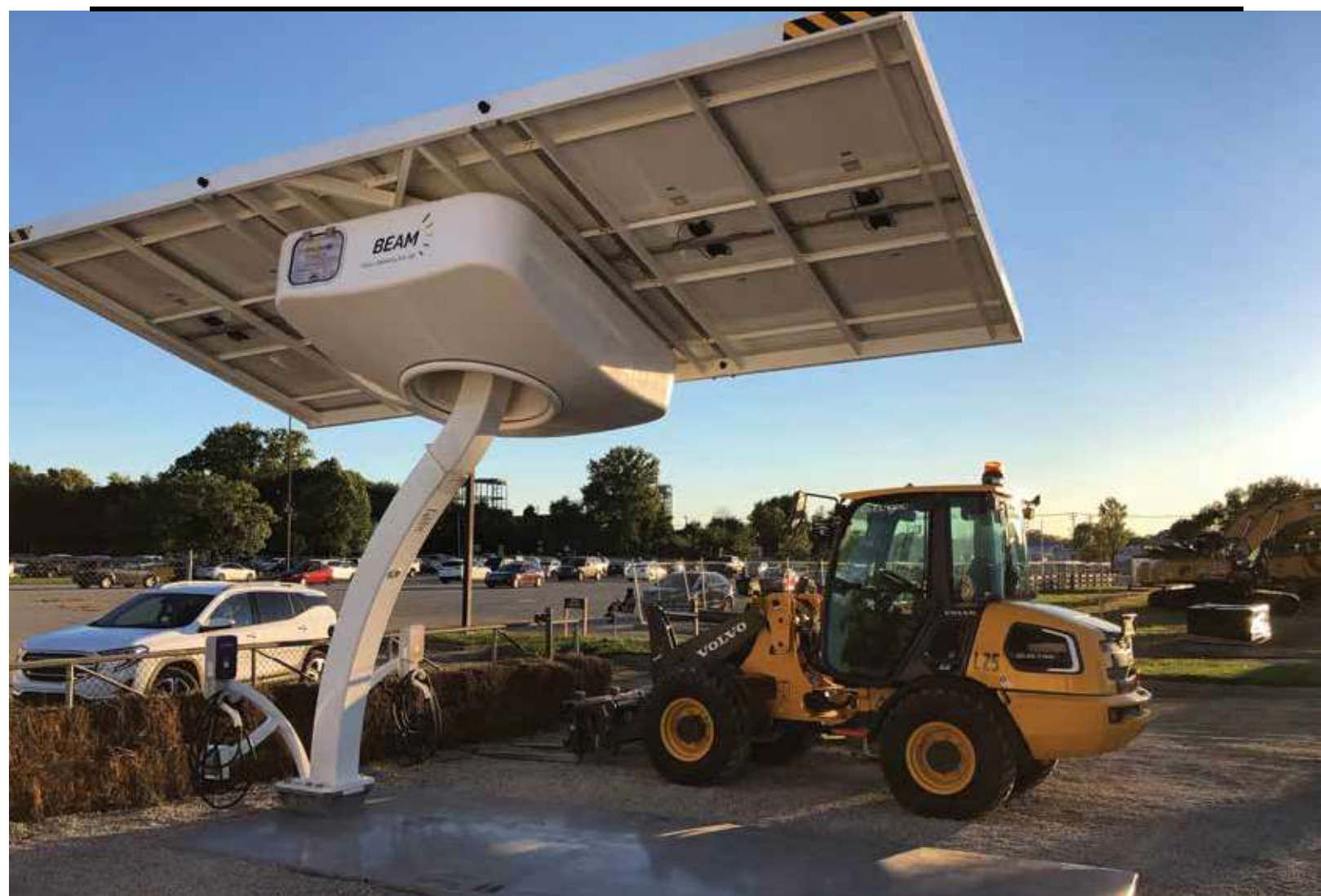
Volvo Electric Compact Wheel Loader Model L25 charging at Beam Station
